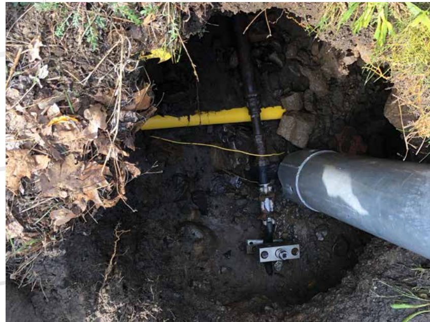
Very critical that we keep a good clean working space around the piping. The vacuum truck has been a great tool in keeping tidiness.
