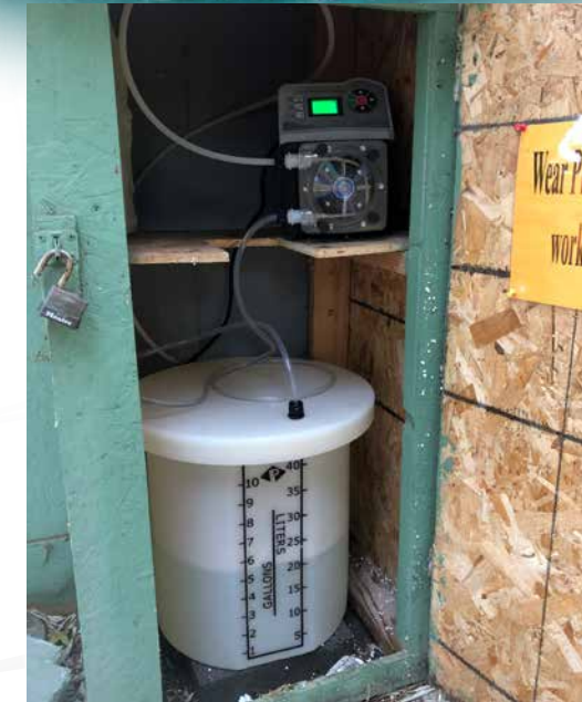
« The District has installed new Chlorine pumps at all sites. The new pumps are peristaltic pumps that replaced the old diaphragm pumps.
